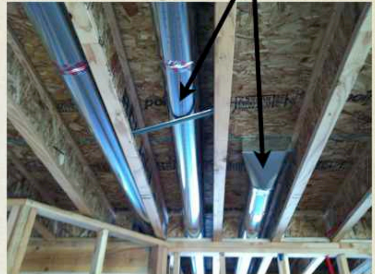
Sheet Metal Ductwork: June 1, 2013 SS Builders
