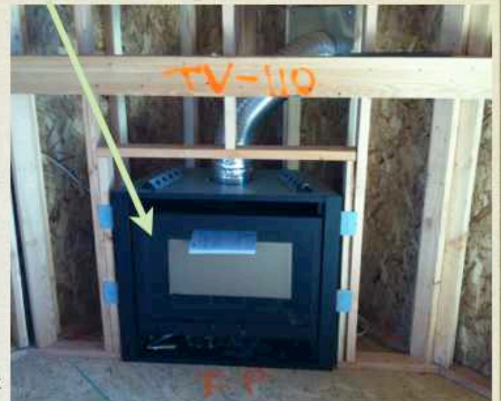
Direct Vent Fireplace : June 1, 2013 SS Builders
