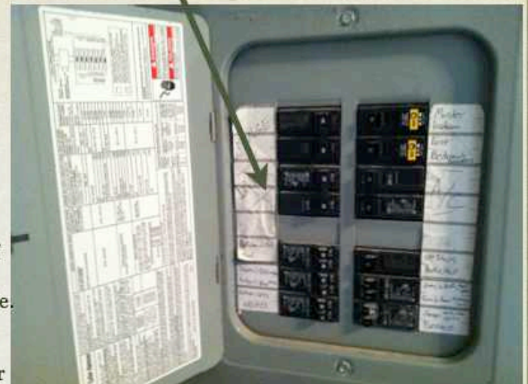
Circuit Breaker: June 1, 2013 SS Builders
